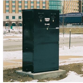
Dubuque, IA Parking lot lighting power and control application. Steel painted black.
