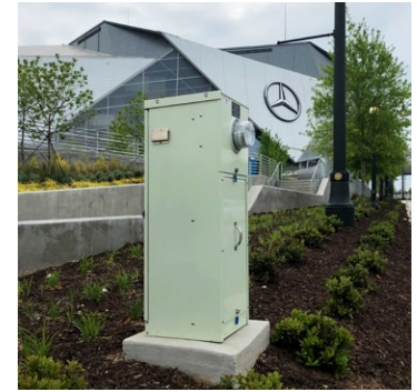
Atlanta, GA Located outside the Atlanta Falcons arena stands a Milbank exposed meter lighting pedestal.
