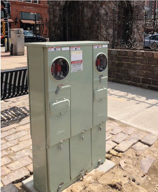
K6342 installation distributes power to cellular repeater.
